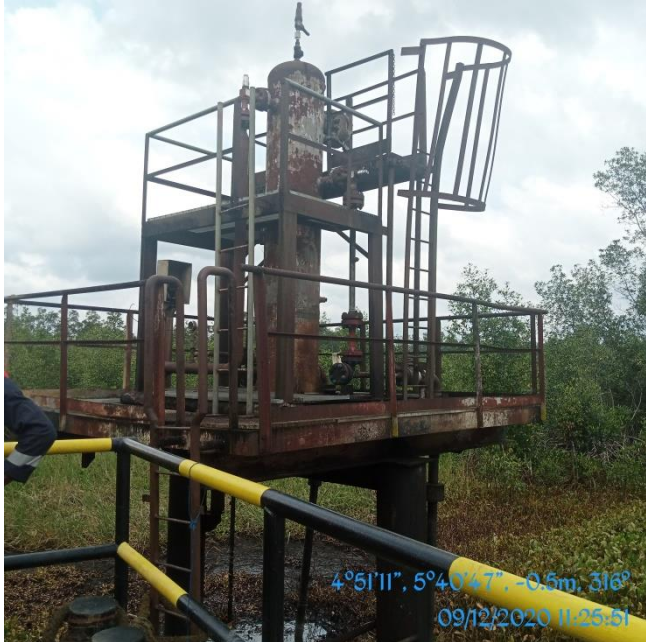
Fig A: Incident Facility (Clough Creek 2 Manifold)
