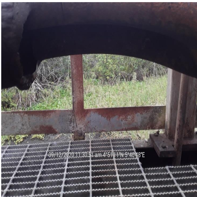
Fig C: Vandalized 4\" Gas F/L
